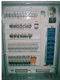
Electrical Parts and Controls
